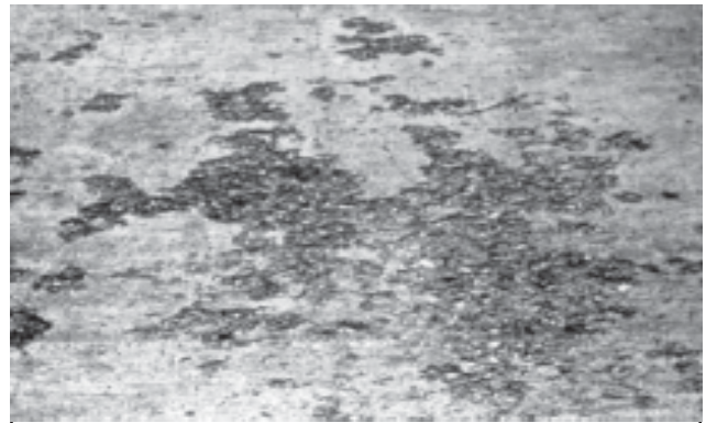
Scaling concrete surface
