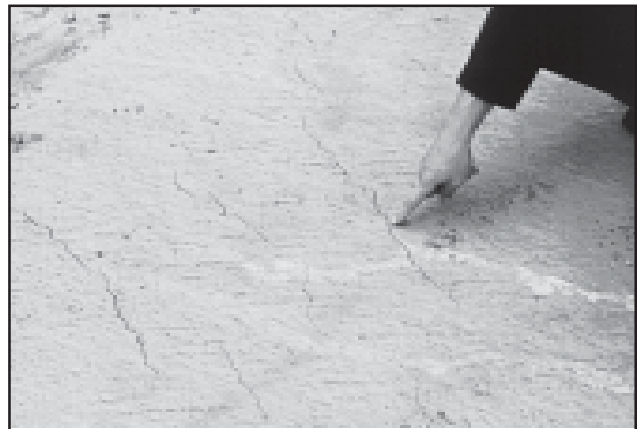
Plastic Shrinkage Cracks
