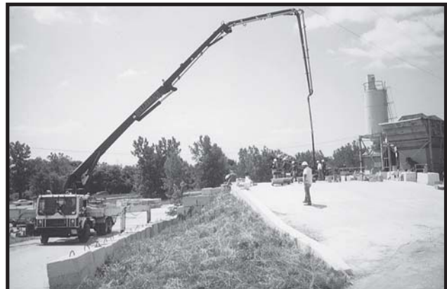
Figure 1: A vertical pump boom configuration can result in loss of entrained air in concrete
